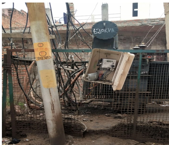
Meter installed at Distribution Transformer under EDD, Chibramau not connected to modem
